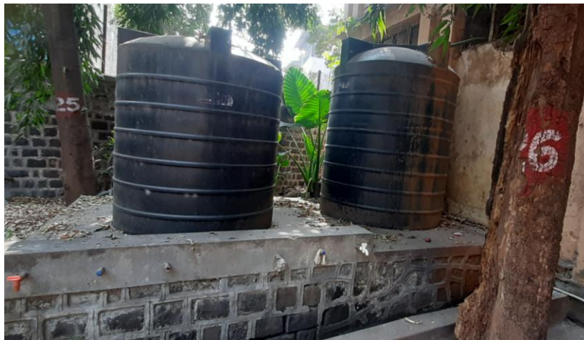
Collection tank for water storage
