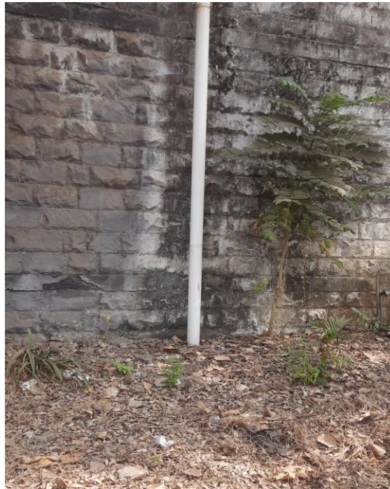
Ground water recharging Pipe
